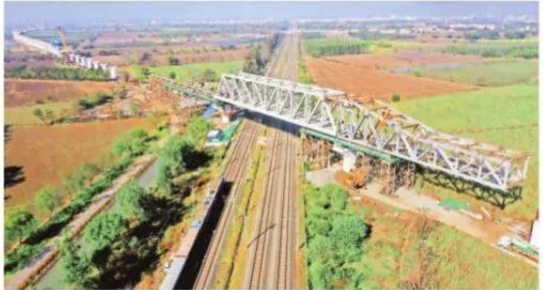
The steel bridge is the sixth of the 17 bridges planned in Gujarat. Express
